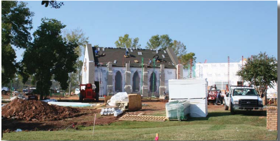
New chapel now under construction at Live Oak Nursing Home in Shreveport
