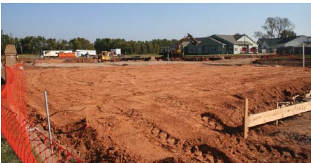
New "neighborhoods" now under construction at The Glen Retirement System in Shreveport.
